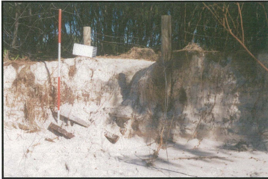
Figure 26. Site ODE2. The slats of this beach track protector were used to estimate the amount of beach recession caused by the April 2000 storm. Photograph was taken three weeks after the storm.
