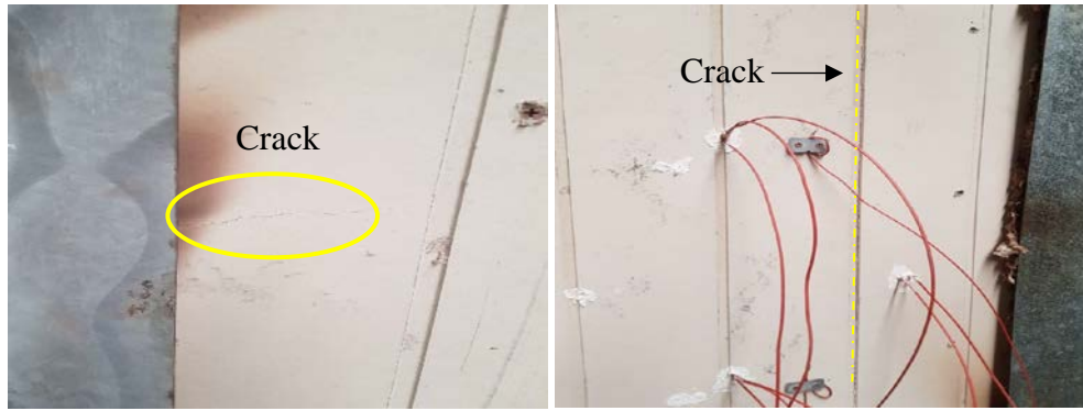
(a) Cracking and discolouration (b) Major crack through vertical joint
