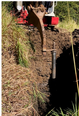
Fig. 1 Insertion of soil sampling tube by the modified adaptor to the excavator's arm
