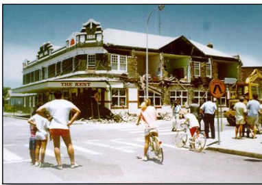
a) Kent hotel after the 1989 Newcastle, NSW earthquake ( M_L 5.6)
