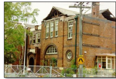
c) The Junction public school after the 1989 Newcastle, NSW earthquake ( M_L 5.6)
