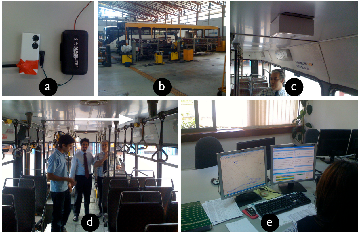
Figure 2: Installation of our system. a: The Gumstix computer (left), along with a 24 to 5 volt converter (right) used to power the Gumstix with the bus' electric circuit. b: a bus being rewired. c: our final installation consisted of a protective plastic case attached to the roof of the cabin. d: the system (indicated with an arrow) is installed near the centre of the main cabin. e: the control centre where real-time data is gathered from the buses' localisation systems and the whole operation is overseen.
