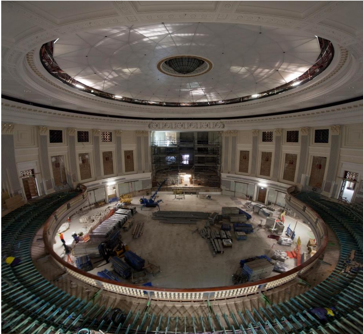
Figure 8: Work completed in the auditorium prior to stage restoration and balcony seating in August of 2012 (Brisbane City Council, 2012)
