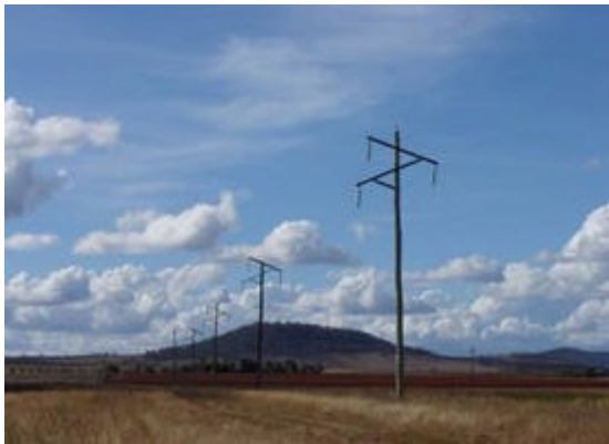
Fig. 1: 110 kV overhead line in typical, flat, isolated area with no adjacent structures.
