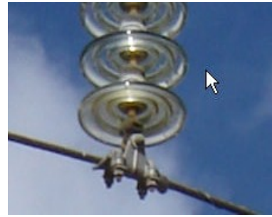
Fig. 9: Cap and pin insulators and a line fitting on the wood pole line. Arrow indicates glass disc insulators.
